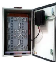
RPST with 200Ah of battery
