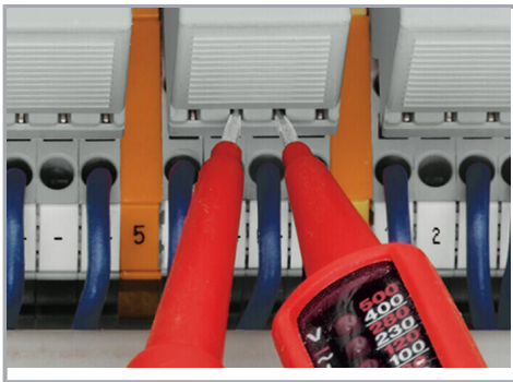
Function testing via touch-proof test slots
